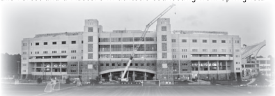
Construction is nearly completed on the west side expansion of Lane Stadium, which will house the SAASS offices.
